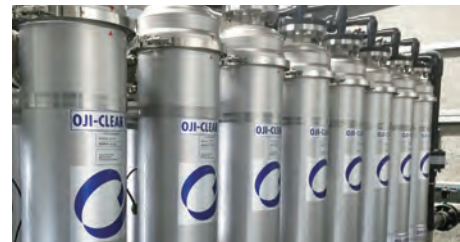
Water treatment system
