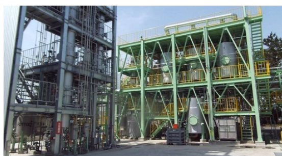
Furfural manufacturing plant (verification plant)
