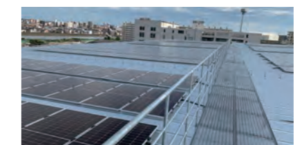
Solar panels at Edogawa Warehouse, Oji Nepia
