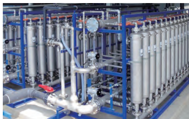
Industrial water production system
