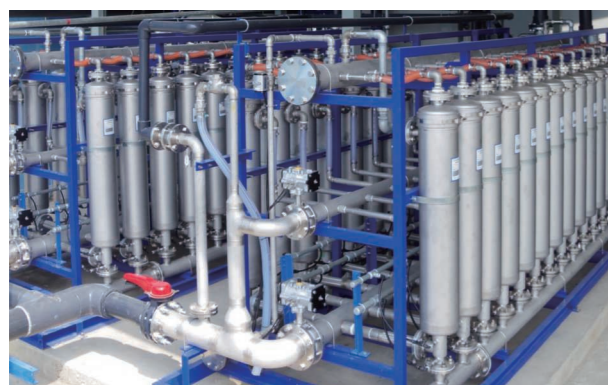
Industrial water production system
