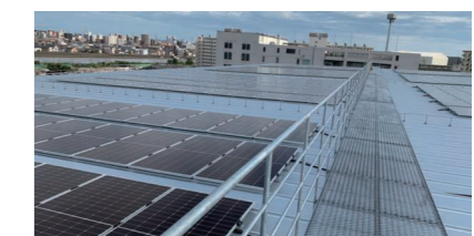
Solar panels at Edogawa Warehouse, Oji Nepia
